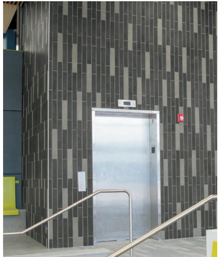
Wall: Main Street | AV214 Gallery Grey | AV215 Boutique Black Designed by: The Miller Hull Partnership
